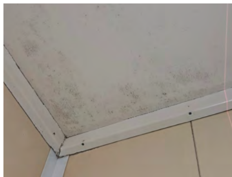
Fuktskader i himling
